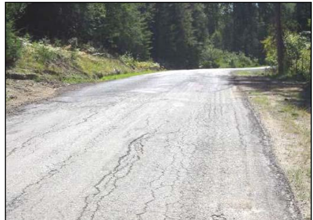
Figure 2. Example of pavement with base problems. (Photo courtesy of the Portland Cement Association (PCA)).
