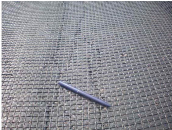
Pic 2. Close-up of Glass grid over cracks
